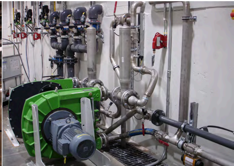
Pumps and piping
