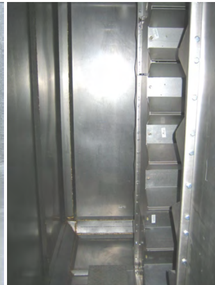
Jet box nozzles from inside
