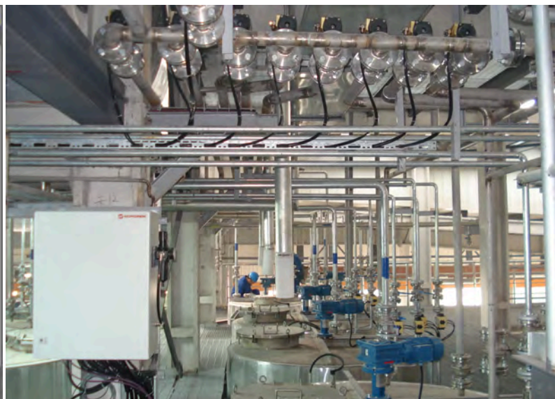
Tanks and piping
