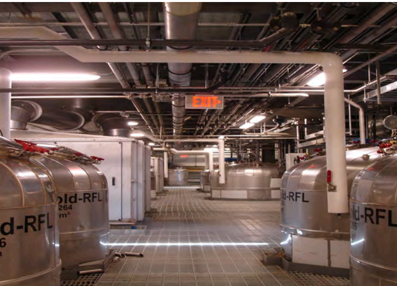
Dip solution hold tanks
